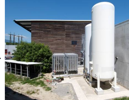
20kW@84K N 2 refrigerator
