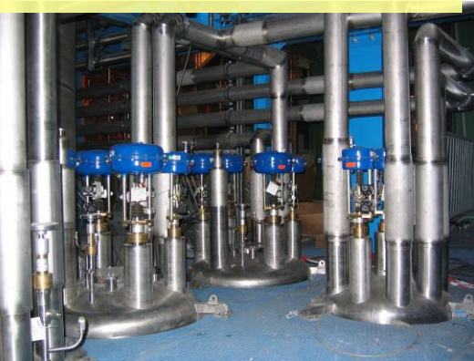
11 distribution valve boxes
