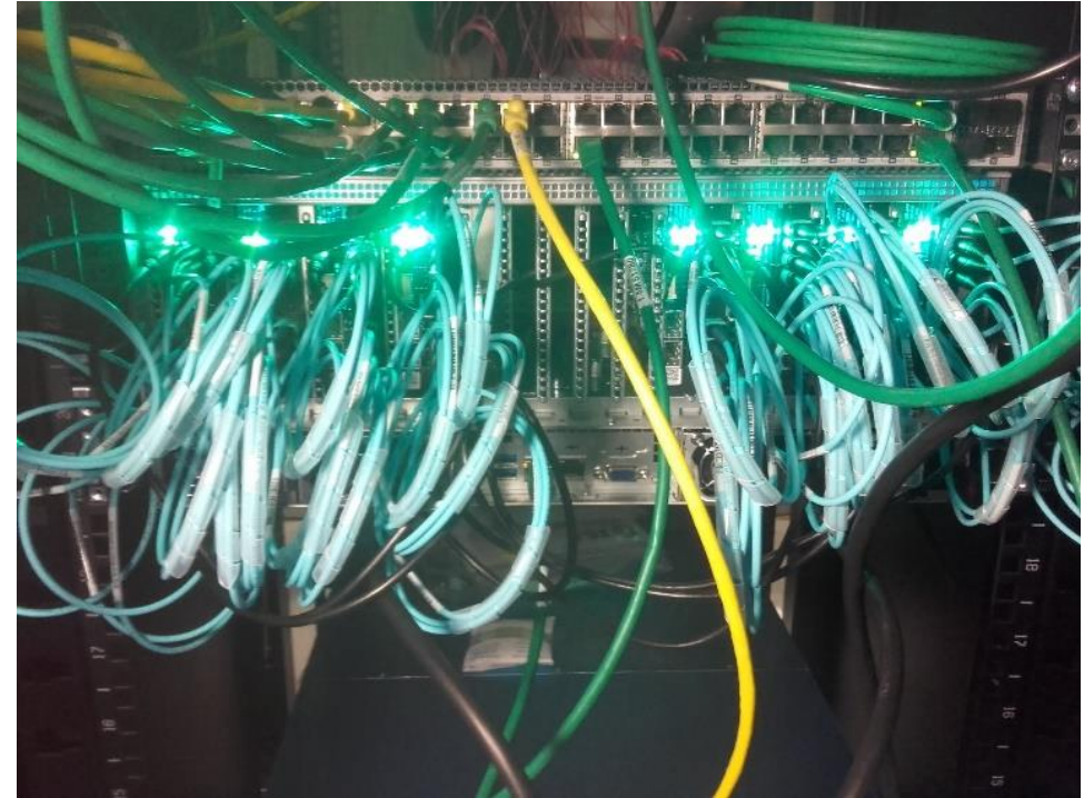
SuperMicro 4029GP-TRT server with 8 TELL40 cards and optical fibres connected
