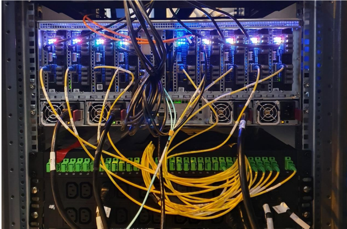
Commissioning backend electronics
