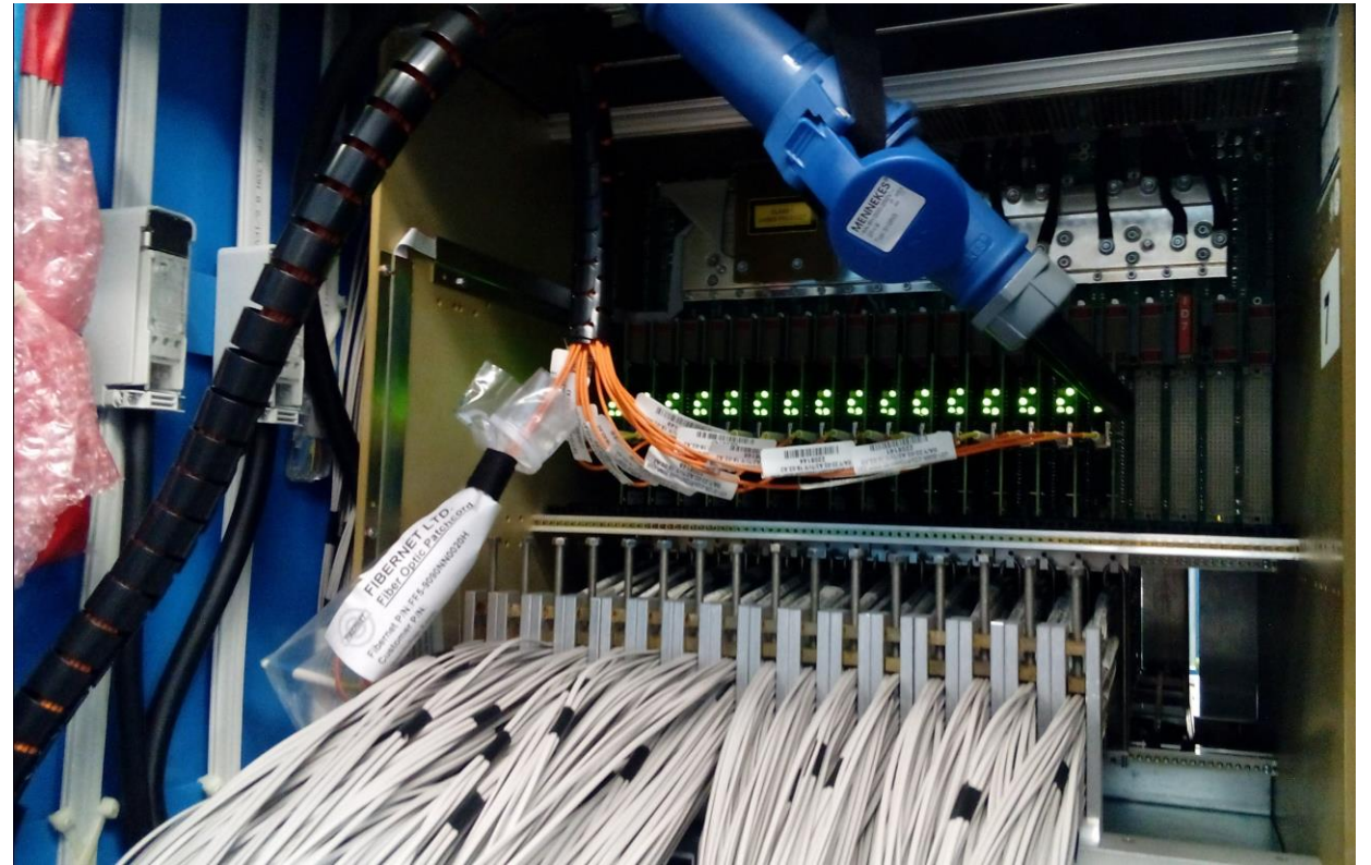
Rear view of the PreProcessor crate
