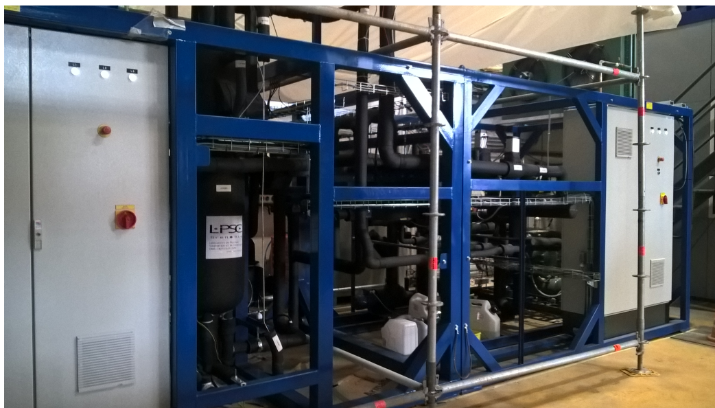
Figure 11.7: CO 2 cooling plant demonstrator located in Building 180 at CERN.
