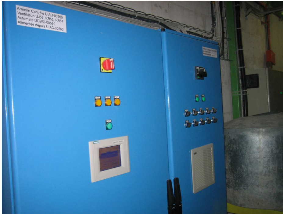
Figure 2. Unit UIAO-00560. Ventilation UJ56, RR53, RR57. Automate UOWC-00560. Power supply from UIAC-00560.
