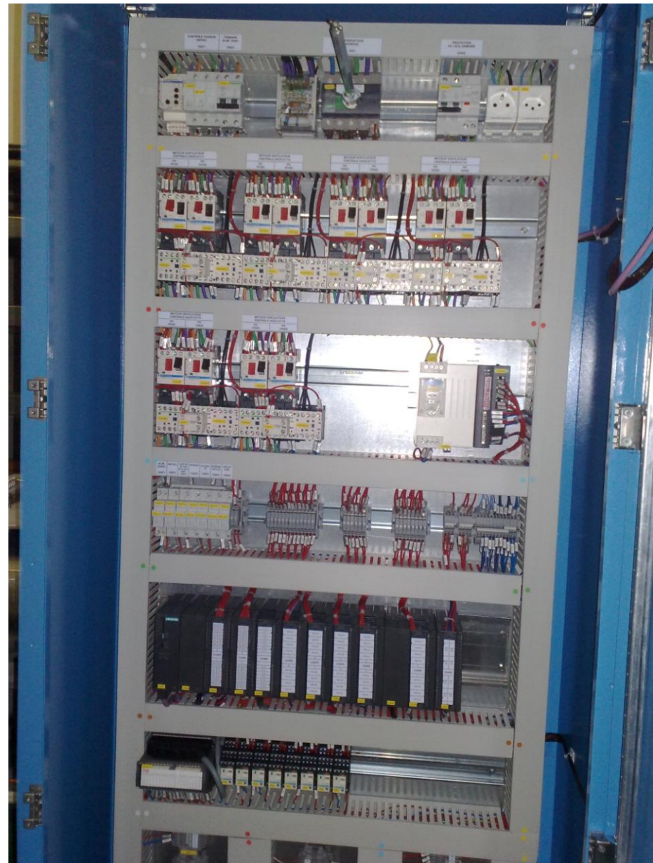
UIAC-770 control rack
