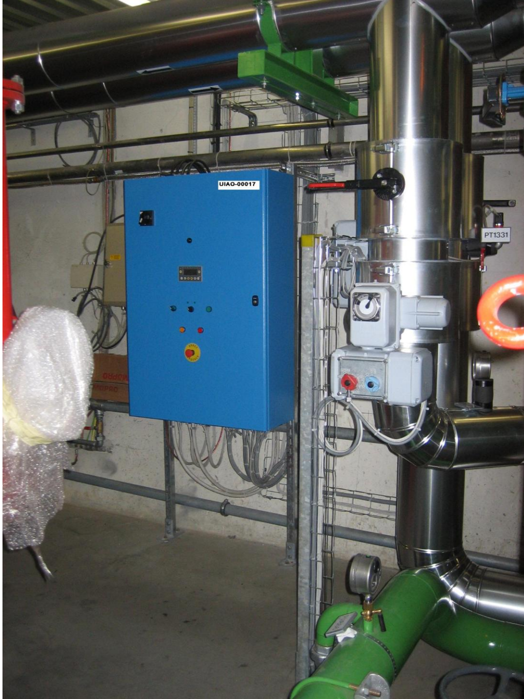
Control Rack UIAO-017
