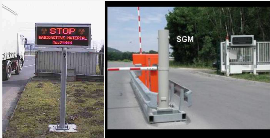
Site Gate Monitor
