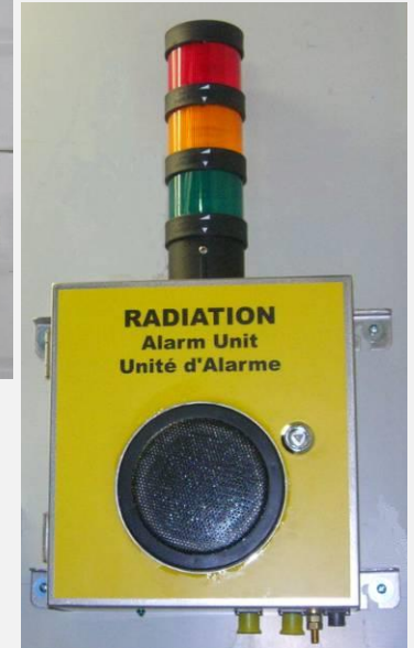
Radiation Alarm Unit (RAMSES)
