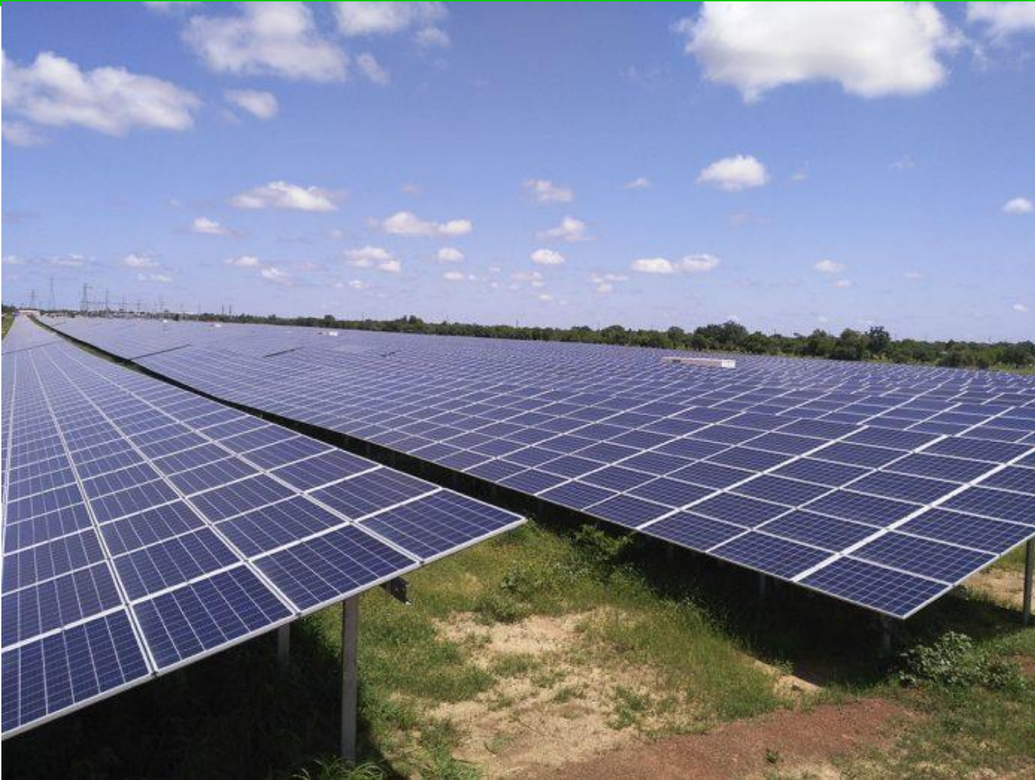
Zagtouli Solar Power Plant in Burkina Faso (33 MW) Major problem: Dust!
