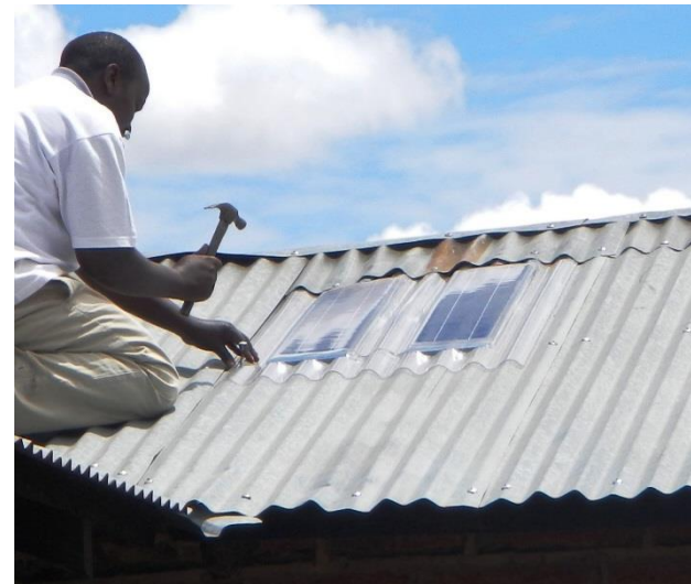
Solamander 36 W photovoltaic panel mounted on a corrugated roof and held in place with nails
