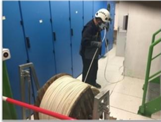
Cabling for new RPC gas racks
