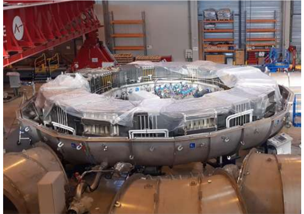
PF6 cold testing preparation
