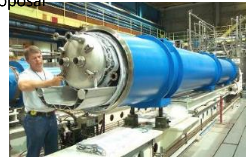
CERN LHC superconducting magnet
