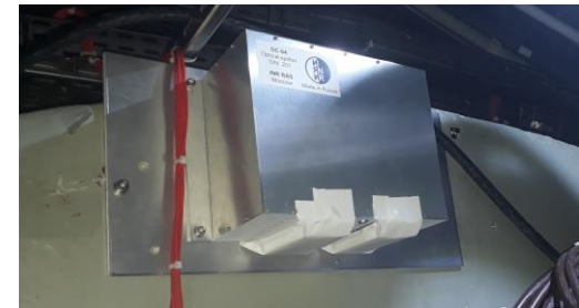
Splitter box (1 out of 2)
