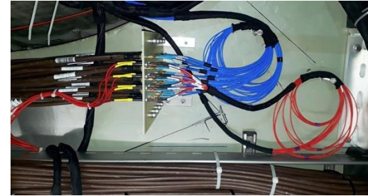
C-side patch panel (1 out of 4)
