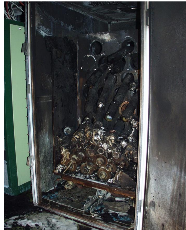
Pulse Forming Network after fire
