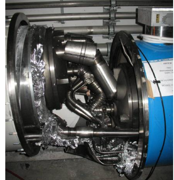
Damage at an LHC interconnect
