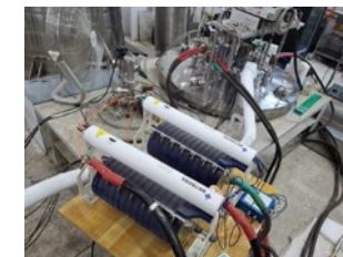
Metrosil Varistor as dump resistor
