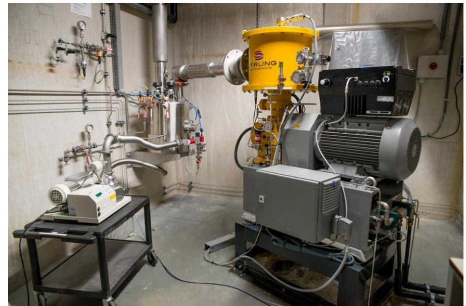
Stirling cryo-cooler and distribution box (1000 W @ 80 K, 20 bar gHe, cryo-fan forced flow)
