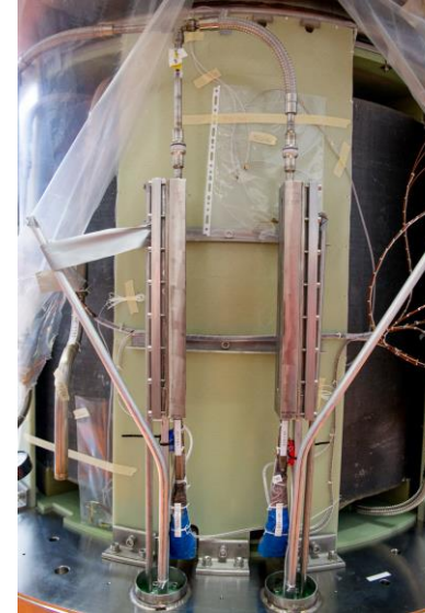
Soft soldered joints bus bar-coil terminals
