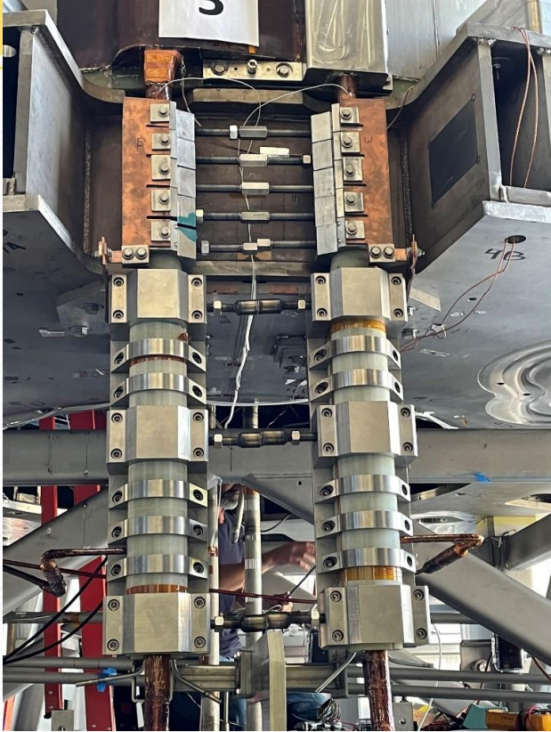
Top left: coil terminal and co-ax joint connection to busbars, as installed
