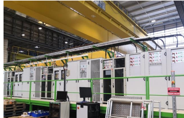
9 Power converters, 3 with energy extraction
