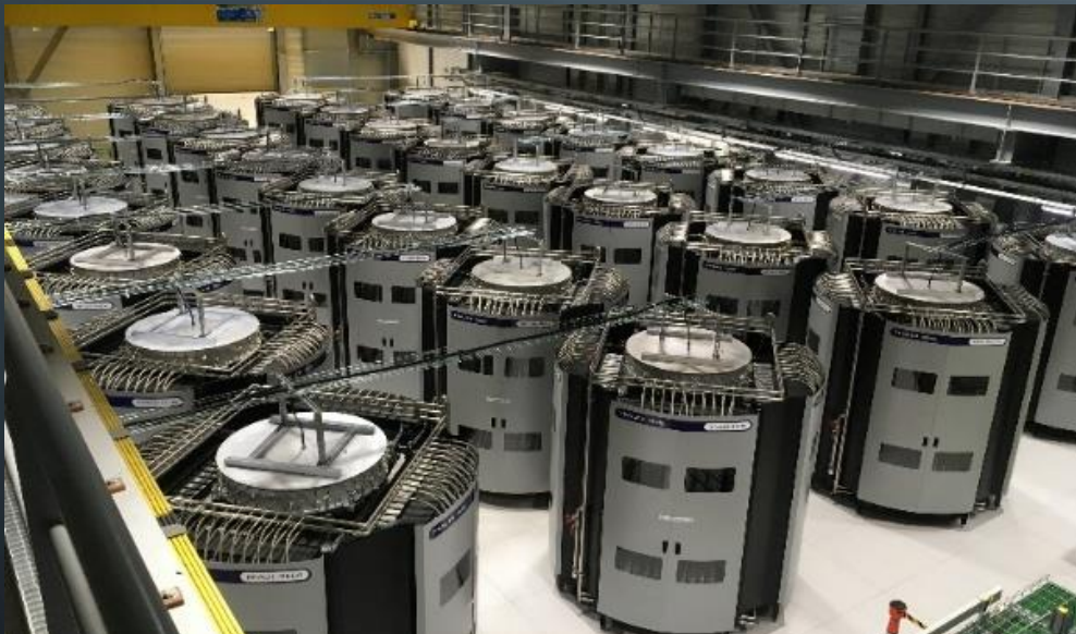
Upstairs: 32 towers of 80 kW each
