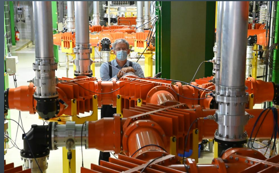
Downstairs: Final combiner stages (16 → 1)
