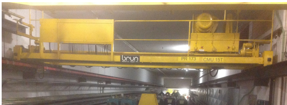
Figure 5.43: Current EOT crane installed in TT4.
