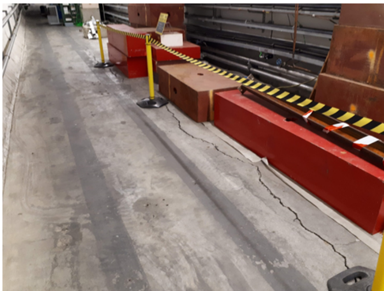
Figure 5.54: TT61 typical cracking in invert.
