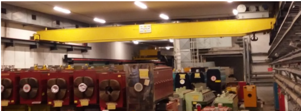
Figure 5.45: Current EOT crane in TT5.
