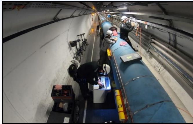
Radiation tolerant electronics Installation
