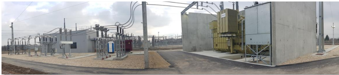
New 400/66kV BE2 sub-station
