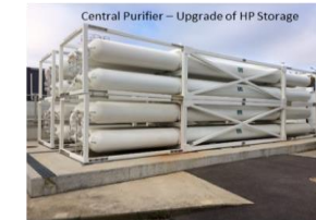
Central Purifier – Upgrade of HP Storage
