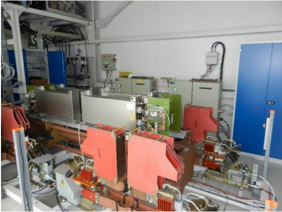
Bdg 377 – 13kA EE systems test area
