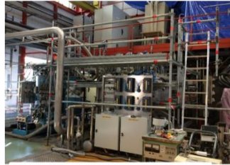
B163 CDS with cold box and control cabinets
