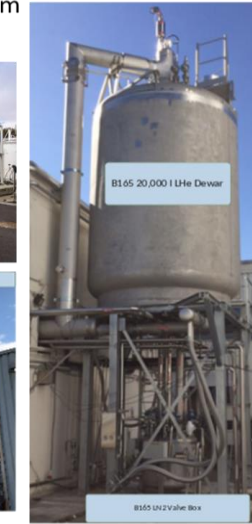
B165 LN2 Valve Box
