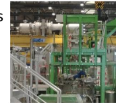
Jumper Connections - installation
