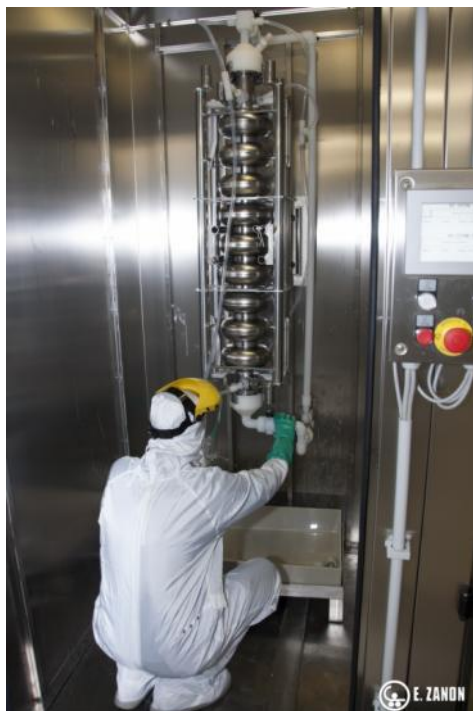
Cabinets for BCP close circuit of the inner / outer cavity surfaces
