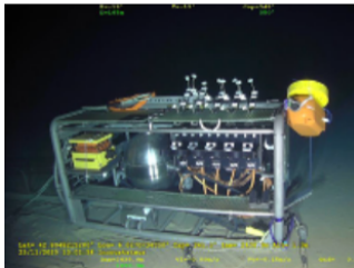
Figure: Junction box
