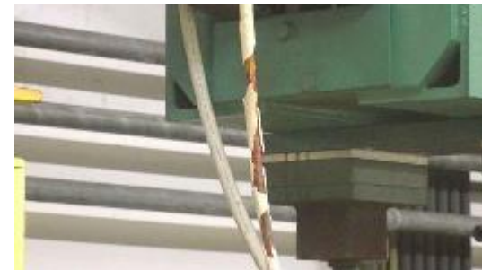
Cabling status inspection
